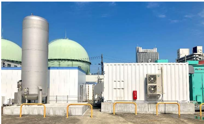
View of AEM water electrolyzer and low pressure hydrogen storage tank
