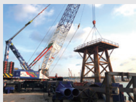
Nong Fab LNG Receiving Terminal
