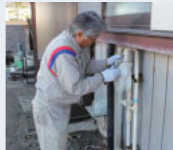
Inspecting a Customer's Gas Meter
