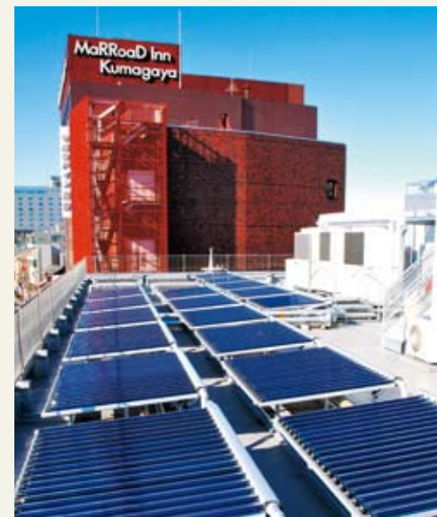
Heat transfer system at the Company's Kumagaya Branch. Solar heat from a solar heat collector (front) installed on the roof of the Company's Kumagaya Branch is transmitted to a nearby hotel (back) through heat transmission lines. This is the first system in Japan that transmits solar heat among private-sector buildings with different owners.
