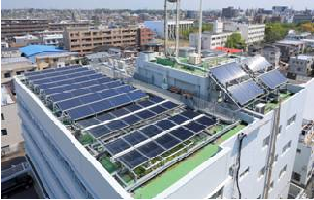
Tokyo Gas Nakahara Building (solar cooling system demonstration plant)
