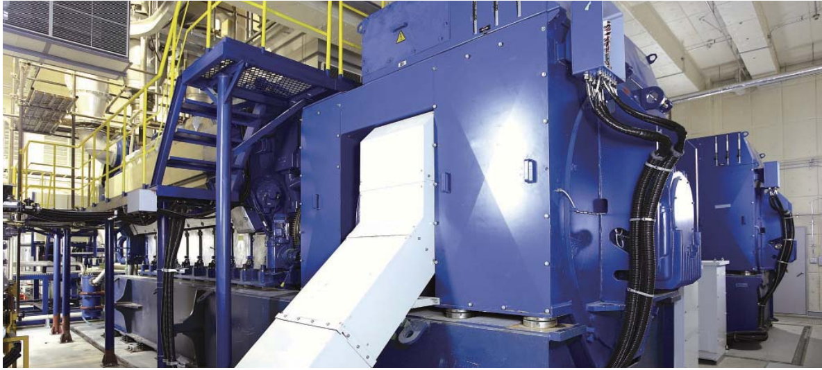
Natural gas cogeneration system using a leading-edge, high-efficiency gas engine (Makuhari District Heating and Cooling Center)
